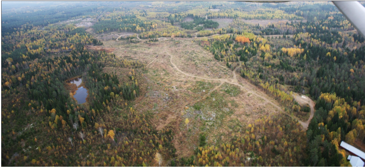
Initial area cleared for laydown and pads, decline excavation will be in centre of cleared area Copyright Markku Mutanen
