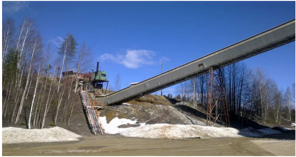
Figure 2: Primary crusher and conveyor belt at the Luikonlahti processing plan
