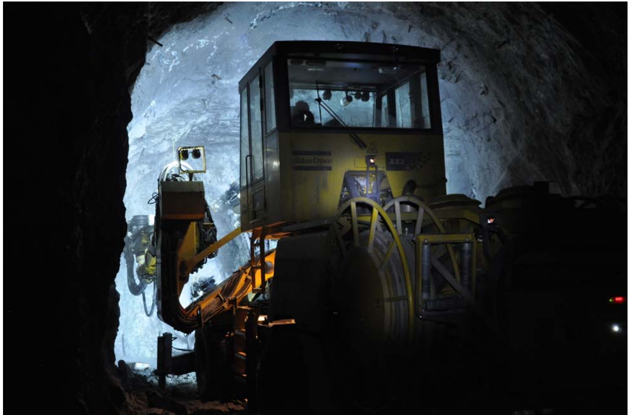
Kylylahti Mine – Contractor YIT's "Jumbo" drilling the decline face. YIT have completed over 1,000 metres of tunnelling
