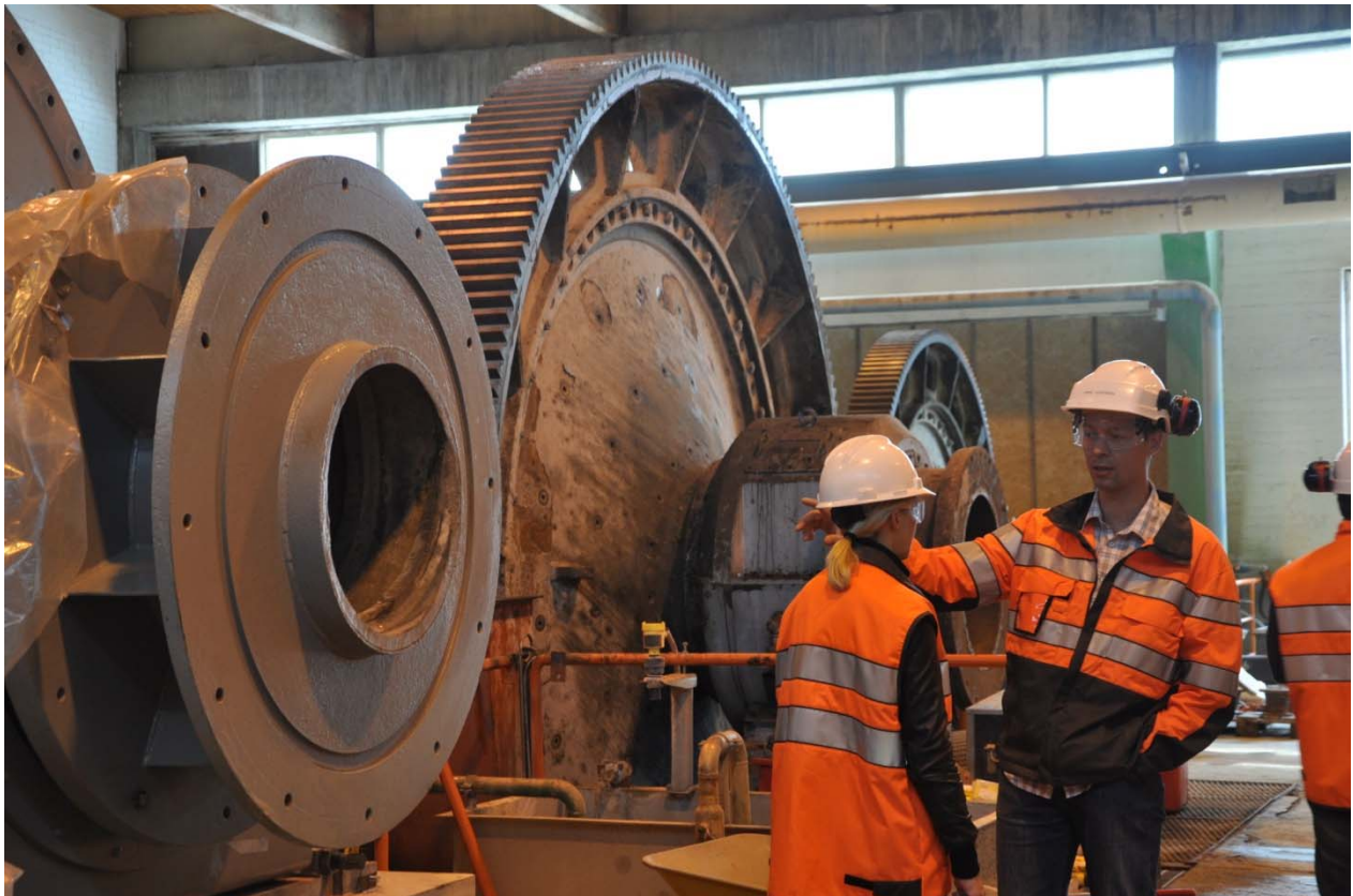
Operations Manager Luikonlahti, Janne Laukkanen, explaining the refurbishment of the processing plant to Flavia Sennhauser from Credit Suisse
