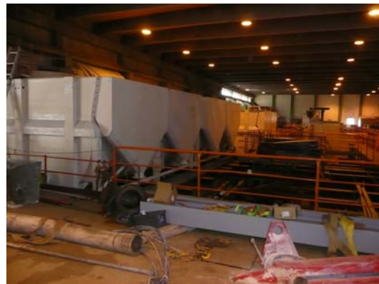
New float cells installed in mill hall
