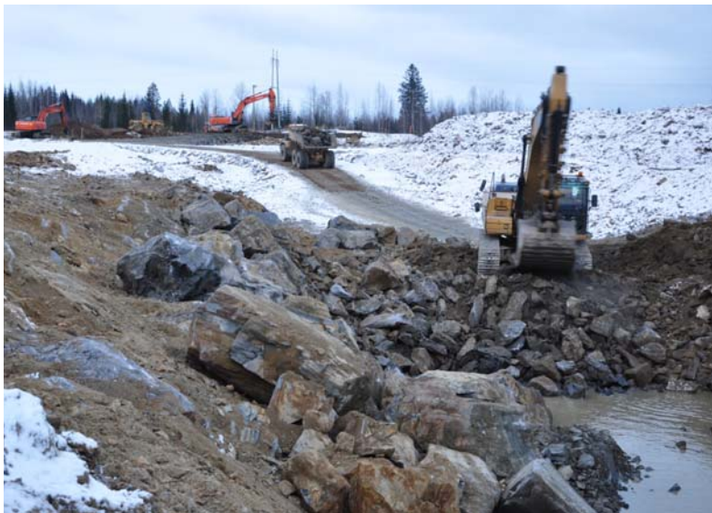
Clearing blasted rock from decline portal excavation Excavators in background working on the office site and installation of power reticulation (Note: Power grid lines on horizon)
